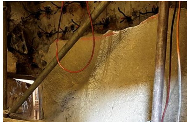
SURGUN 50SCZ EXTRA Panel shown in Riser duct after 12 months of service
